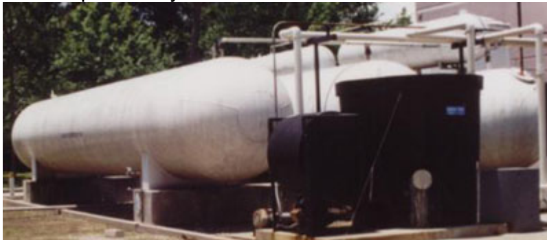
Photo 7 - Delta Cooling Tower with Helium Vessels in Background
