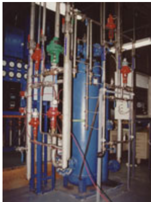
Photo 3 - Gas Management Rack
