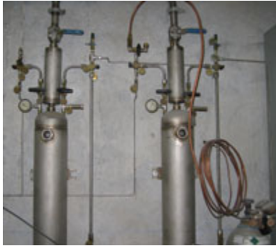
Photo 6 - Compressor Oil Purifier
